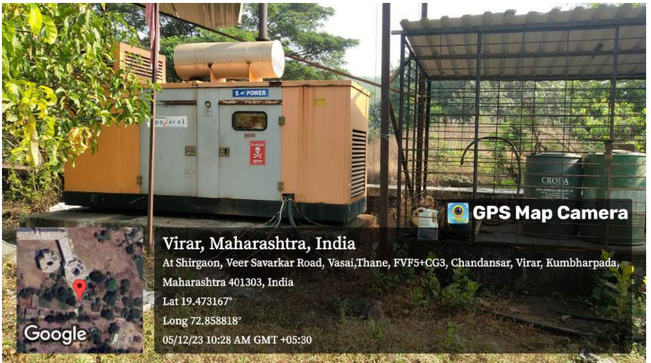
Generator in campus
